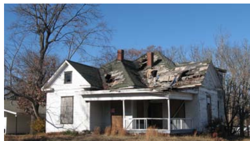
No overlay, no protection, no future. Without local ordinance districts or demolition-by-neglect provisions, this can be the result (4200 W. 16 th Street).
