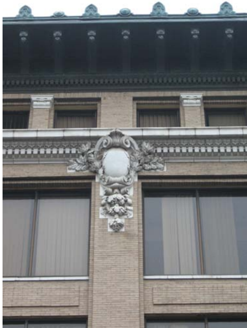
Vacant space in downtown historic buildings offers potential for loft apartments and condominiums (320-322 S. Main Street).
