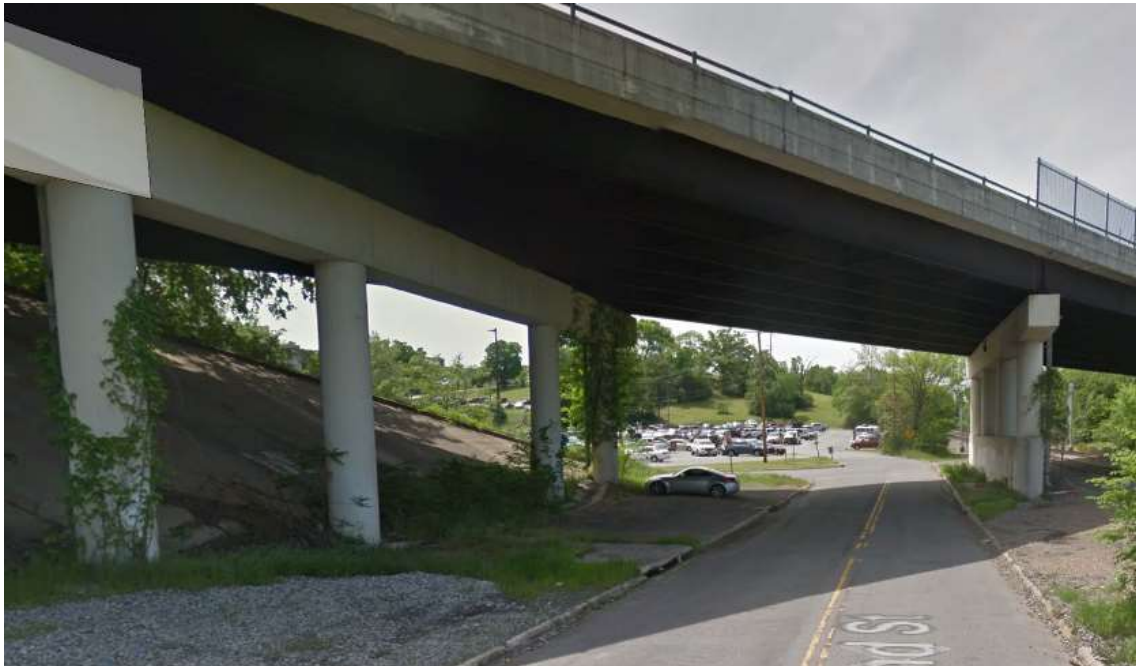
Figure 39. Getting the Corridor under 3 rd St., between the two 3 rd St. Bridge support pillars that surround 2 nd St., is another challenge. Note the drains on the left side of 2 nd St.
