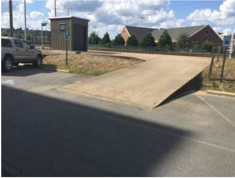
Figure 17. One of two ramps that extends into the parking lot (Fig. 14, left center). The proposed trail route runs closer to the building to avoid these ramps.
