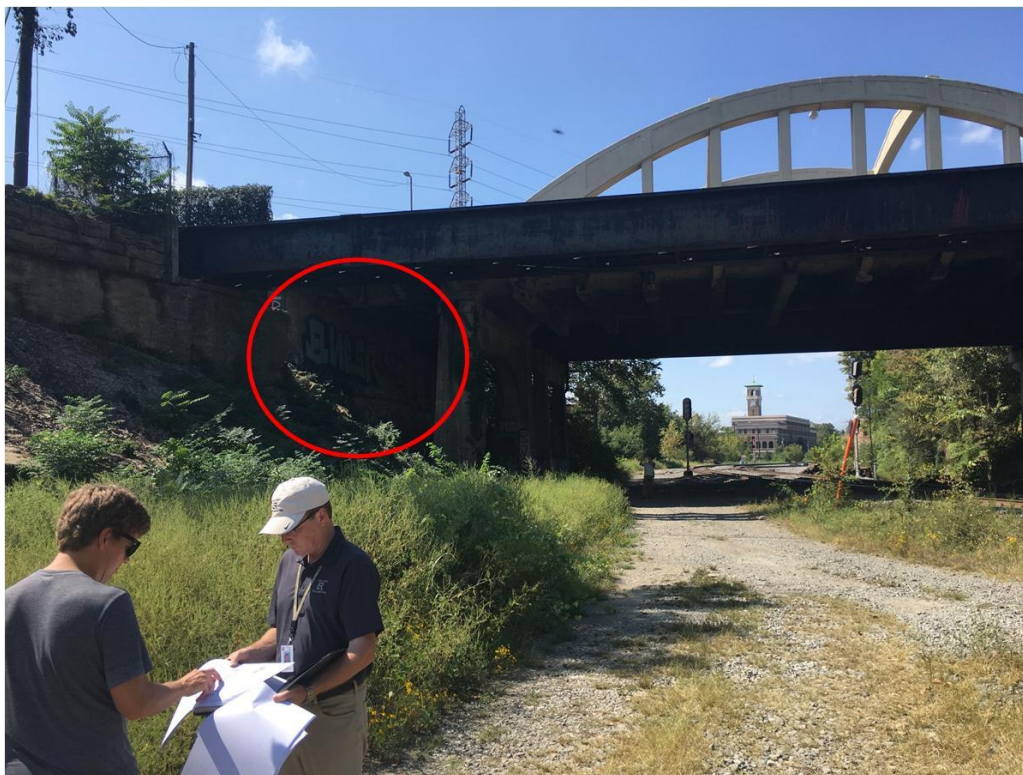
Figure 2. A trail between the eastern LaHarpe Bridge abutment and the eastern LaHarpe pillars (red circle) would give every possible allowance to Union Pacific safety and expansion concerns.
