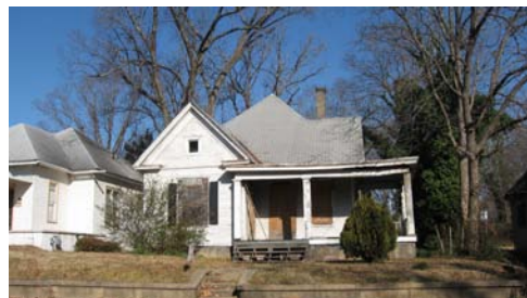
The use of Urban Homesteading and Revolving Fund programs could assist in reversing vacancy and abandonment (3412 W. 13 th Street).
