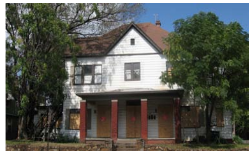
Demolition by neglect provisions would require owners of vacant properties to maintain houses to minimum standards (420 E. 9 th Street).
