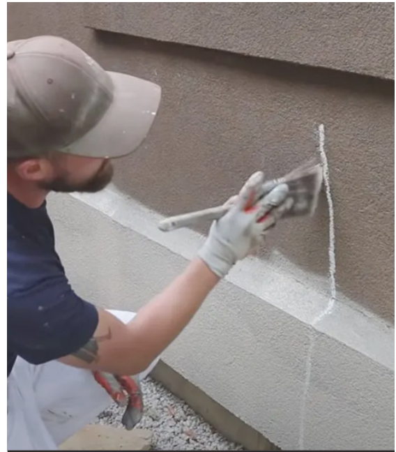
Use paint or limewash to repair small cracks in historic stucco. © Tape University
