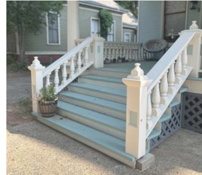
Wood steps match the porch floor at 514 E 8th St.
