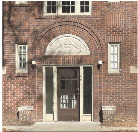
Repair deteriorated or missing mortar joints in masonry door surrounds to prevent water infiltration, 406 E 7th St.
