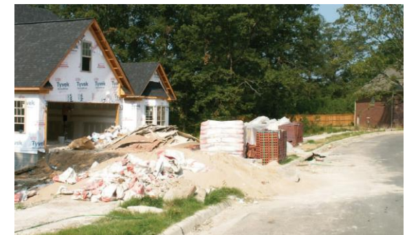
Example of a poorly maintained construction site. Note the sand piled into the street and un-contained debris and trash.
