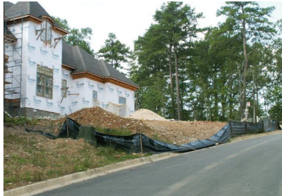
This silt fence is not being maintained properly. It should be re-installed to contain storm water run off.
